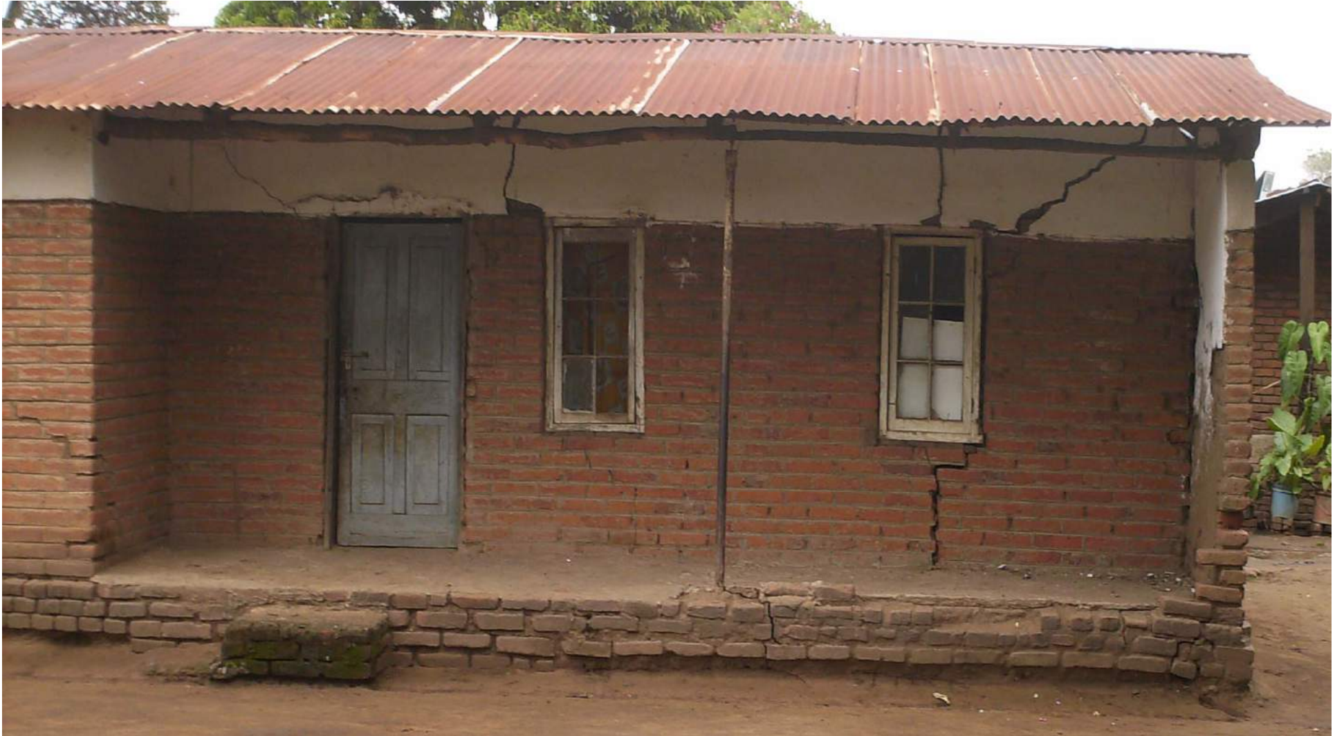
Figure 6: 2009 Karonga earthquake affected building (magnitude 6)
