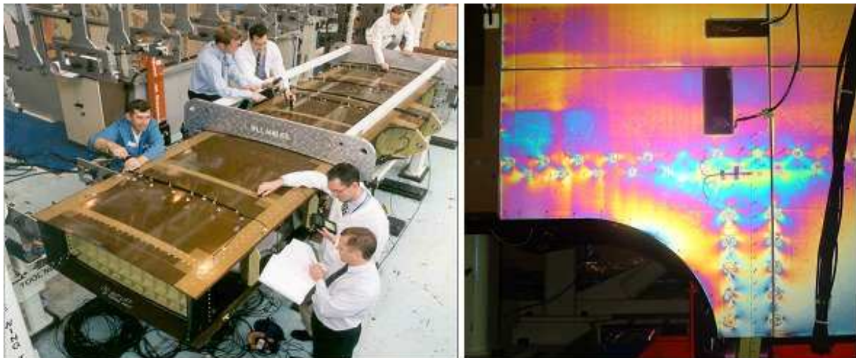
Figure 1: HLIE under construction (left); photoelastic image of skin at pylon area under load (right)
