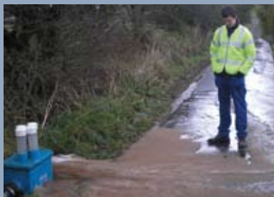
Ice pig leaving a mains water pipe.. Yes this is the water you drink!! But now that the ice pig has cleaned out the pipe it's a lot better
